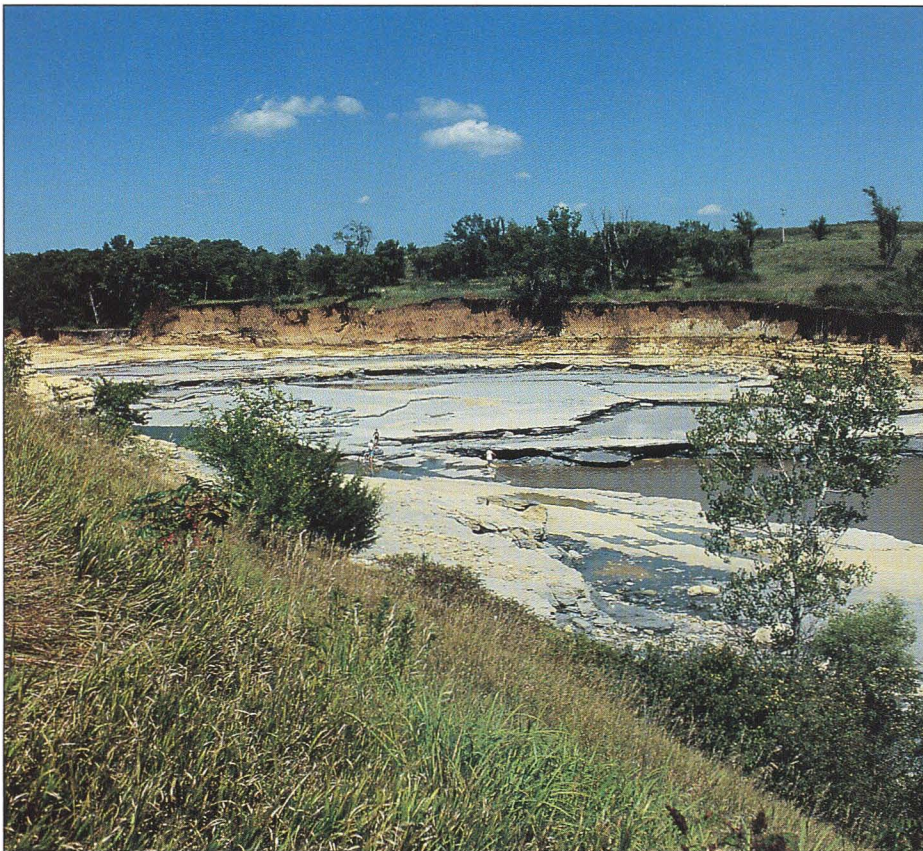
The force of flood waters are never more evident than by the gorge carved here by water released at the emergency spillway at Tuttle Creek Reservoir.
